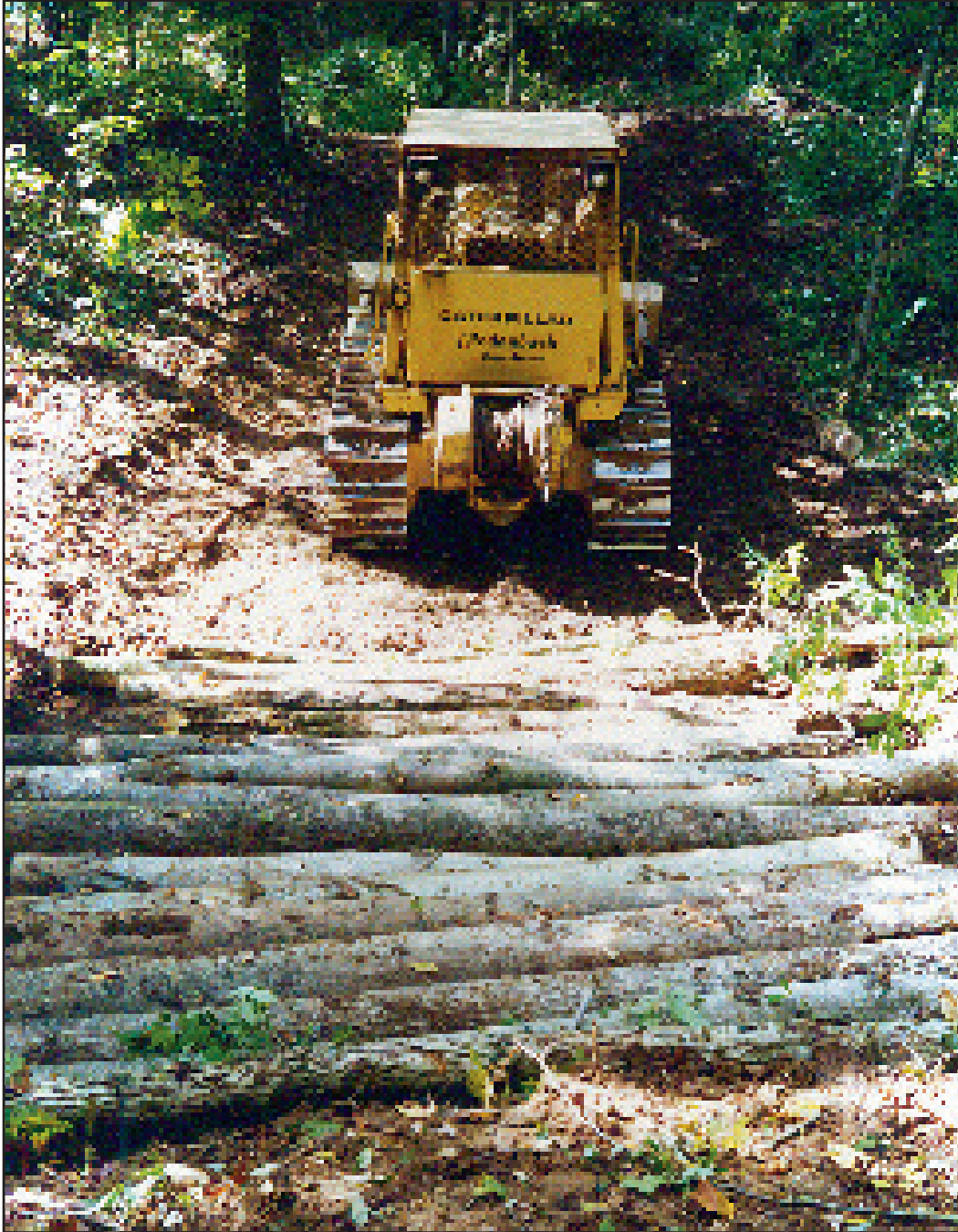
Figure 23B. Pole crossing.
