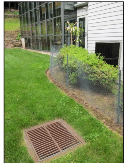
Well maintained residential dry well
